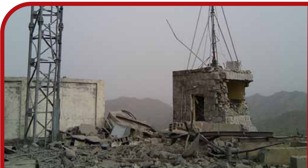
Communication station – Saqain- Saada - bombed in 25/4/2015
