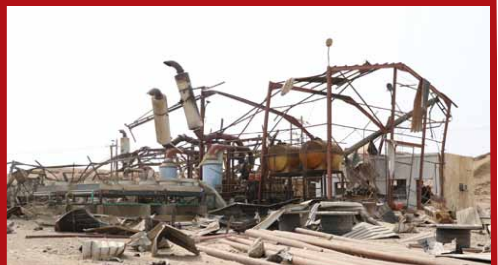
power station Al-lohaia –Al-Hodida, bombed in 23/8/2015
