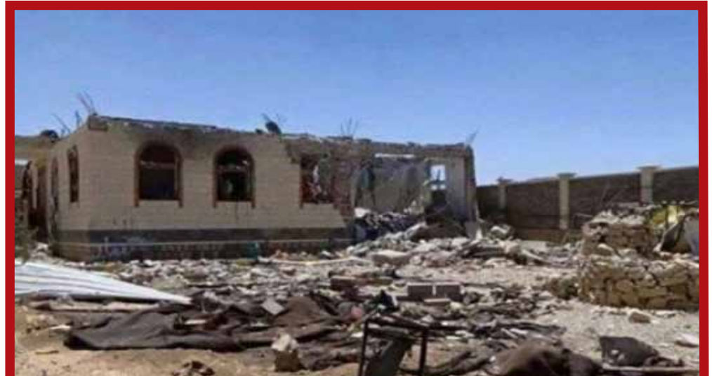
Al-Masira Channel building - bombed in 9.5.2015
