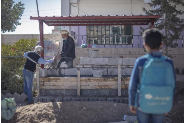
©UNICEF Yemen/2019 UNICEF supports construction of WASH facilities in schools. Photo was taken in the Sana'a governorate.
